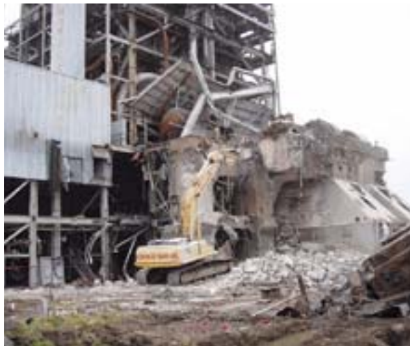
This project includes demolition and remediation of more than 30 facilities, including three generating units. The largest generating unit was imploded on January 13, 2007.
