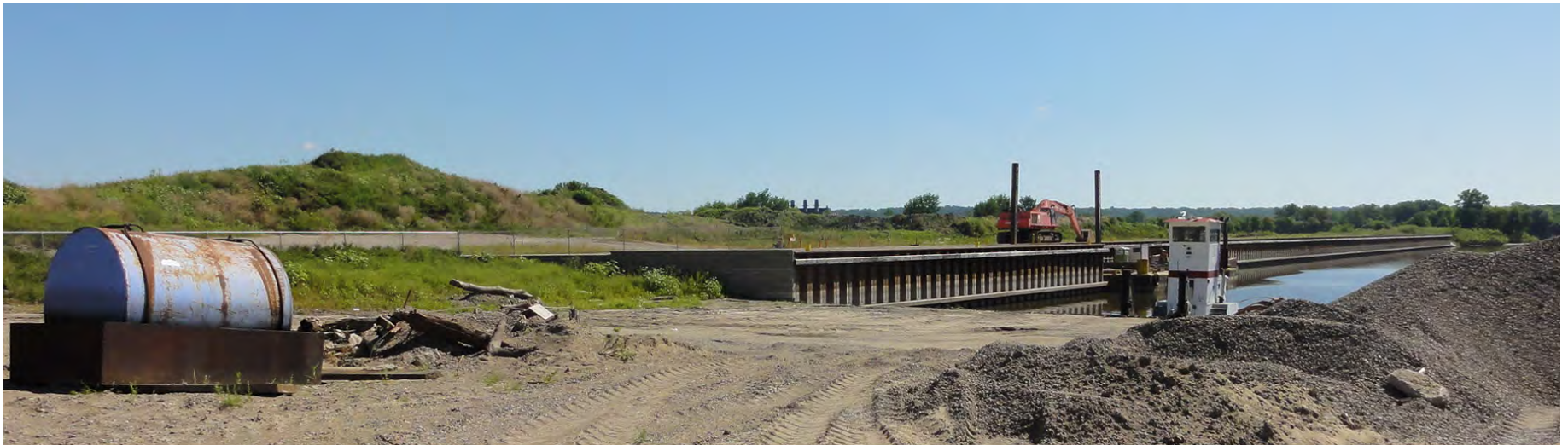
The Port Authority has recently completed a new dockwall along the Harbor split
